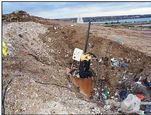
Photo 12: Poorly installed control panel – too close to potential release point of landfill gas
