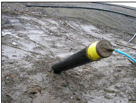
Photo 23: Poor Design - bucket used as a head works and sealed with tape
