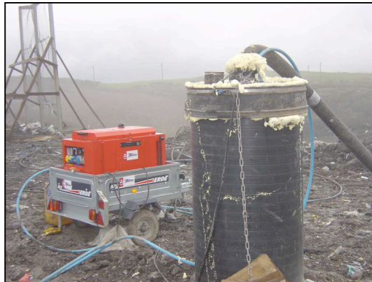
Photo 1: Generator located within a zone 2
