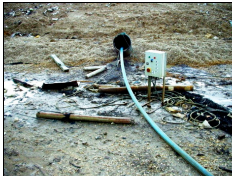
Photo 18: Open side riser producing a large potentially explosive atmosphere
