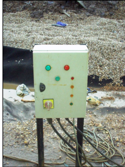
Photo 19: Control panel showing signs of corrosion
