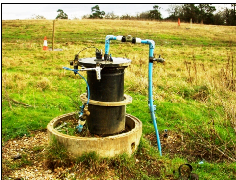
Photo 22: Blanking plate on the leachate chamber not secured
