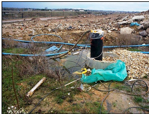
Photo 11: No headworks installed on leachate chamber
