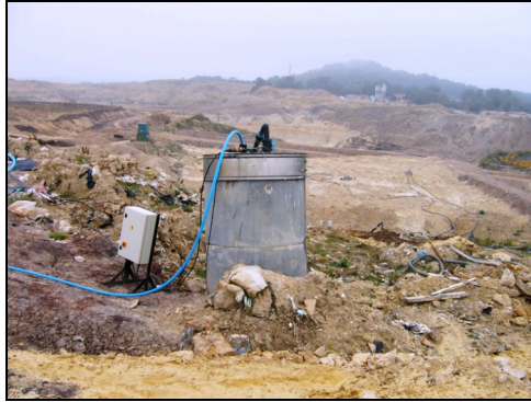
Photo 16: Control panel installed too close to leachate chamber
