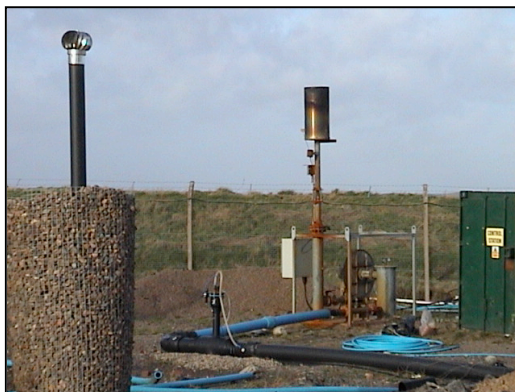
Photo 8: Flare located too close to a vent
