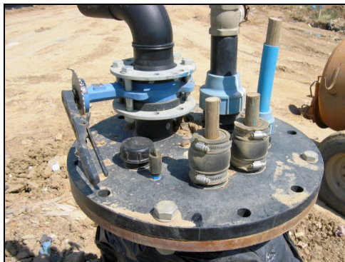
Photo 14: Poor standards of installation
