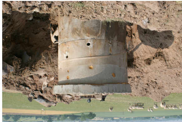
Photo 7: Excavation with the potential for landfill gas to accumulate
