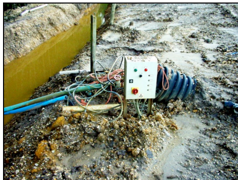
Photo 15: Poor standards of installation – control panel Located within zoned area
