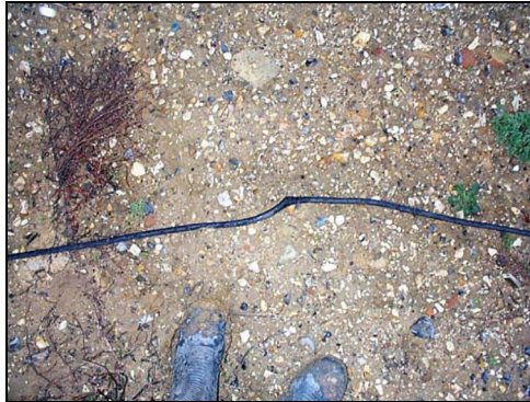
Photo 10: Badly repaired cable joint using electrical tape
