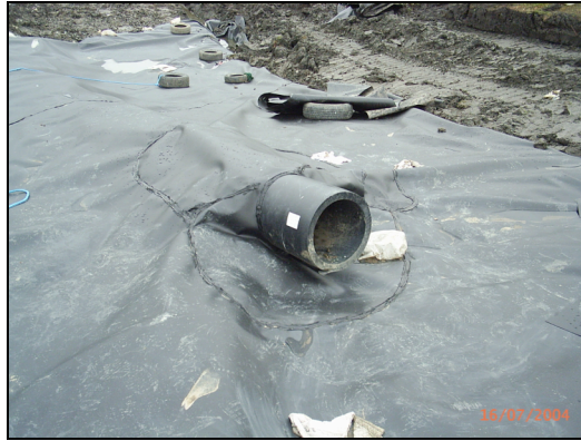
Photo 4: Boot and skirt around a leachate well
