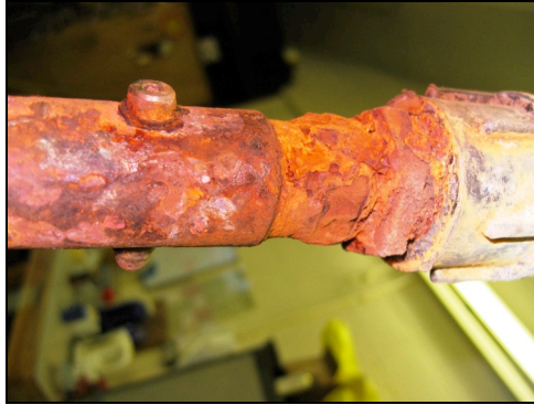
Photo 13: Lack of maintenance – excessive corrosion of borehole pump.
