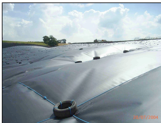
Photo 2: 'Ballooning' due to landfill gas collecting under geo-membrane
