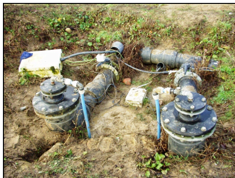
Photo 21: Poor installation - control panels left on the ground within zoned areas
