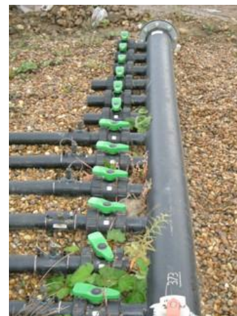
Manifold direct on ground (not recommended for permanent installations)
