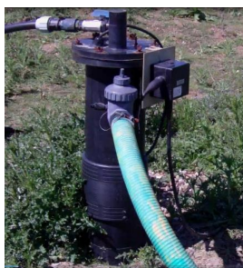
Wellhead with electric leachate pump
