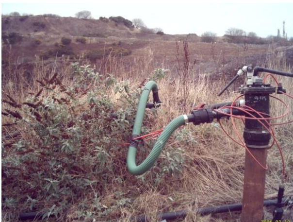
Hose tied up with air line and forming condensate trap
