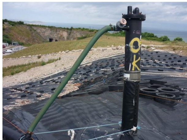
Flexible hose too short
