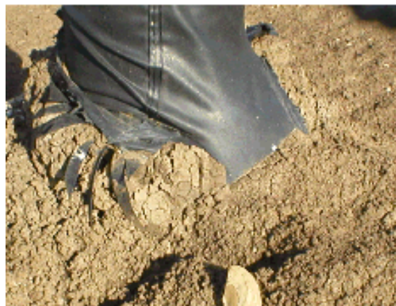
Damaged top hat seal
