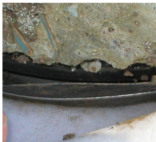
Damaged seal detail
