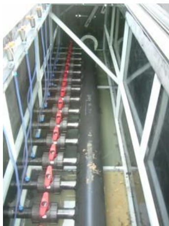
Manifold in a chamber
