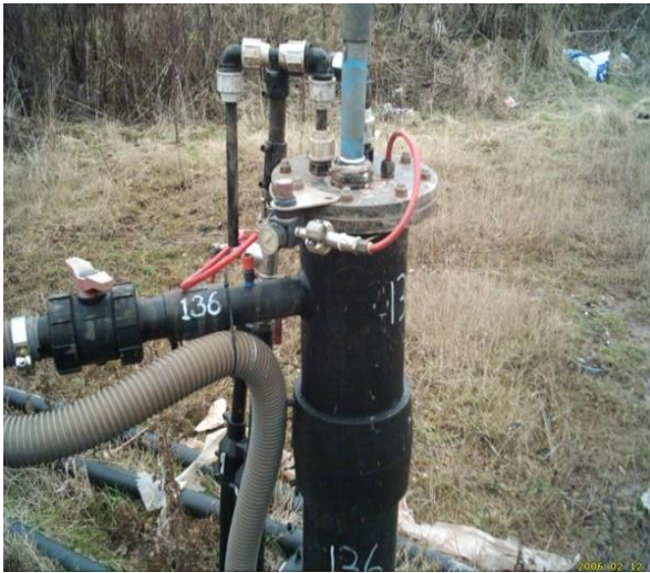
Hose tied to outlet. Uphill path could create condensate trap
