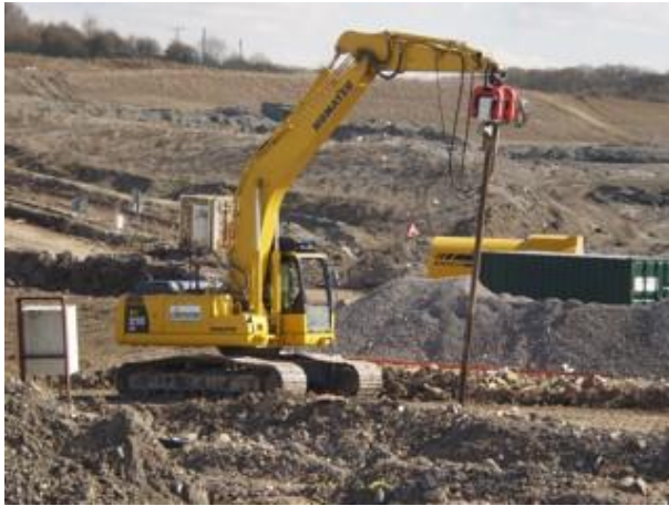
Void made with impact drill
