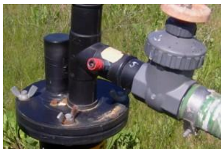
Wellhead with valve and sample point
