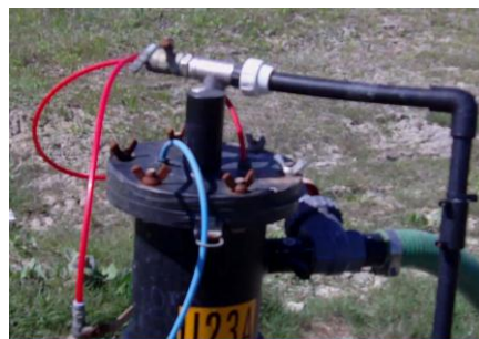
Wellhead with sample point and air driven leachate pump
