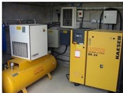
Figure 7.21: Air Compressor with Refrigerant Dryer
