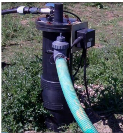
Figure 7.17: Electric Pumped Wellhead
